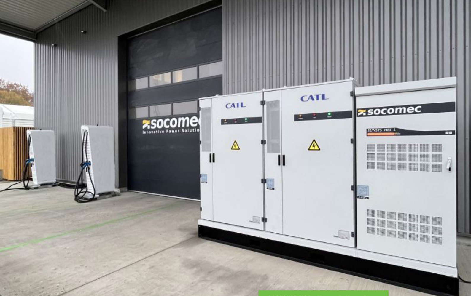
© SOCOMEC, ESS Test Platform, Nordhouse, France
