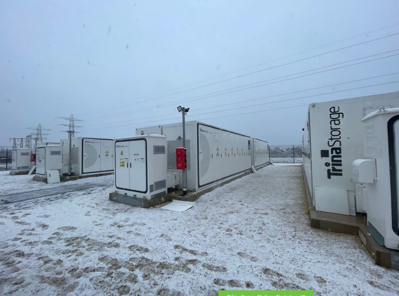
© Trina Storage, Tilt Farm, Birmingham, UK
