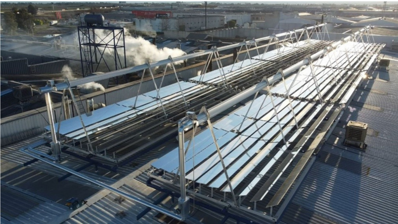
A 30 MW CST Plant in a brewery in Spain, covers 55% of the heat demand with the remaining 45% covered with biomass. © Protermosolar
